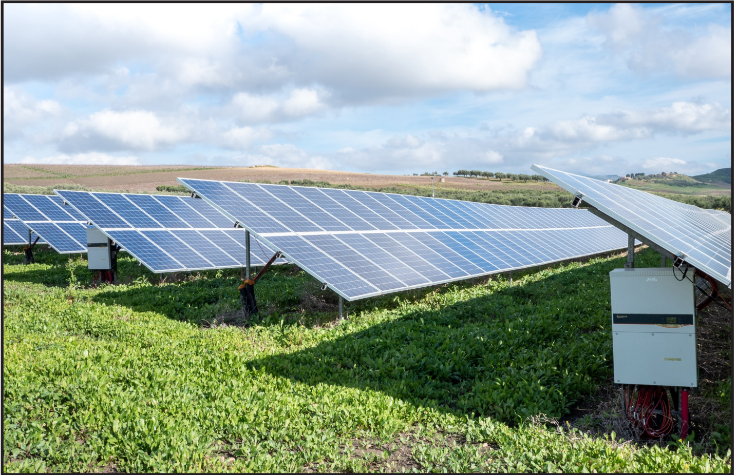
Solar Panels located in Italy Photo via Sungrow EMEA on Upsplash
